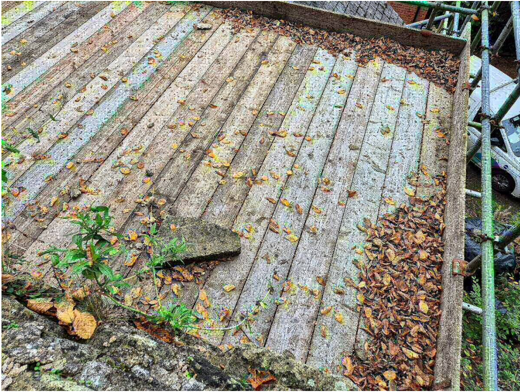
Photograph 3 – Debris on the scaffolding
