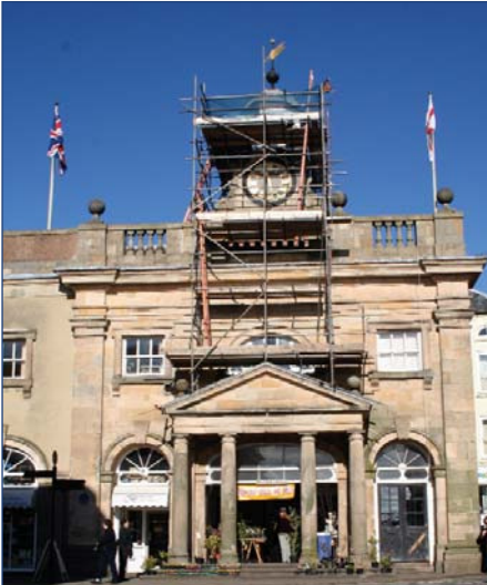
The Buttercross, a Grade 1 Listing Building owned by the Council, needs major repairs. Phase One is urgent work on the cupola.
