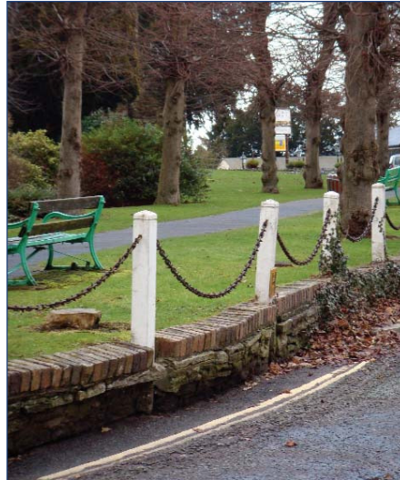
Sections of the retaining wall in Dinham Gardens are collapsing and damaging the fence. Repair work is clearly needed.
