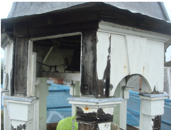
Current condition of the cupola on the Buttercross
